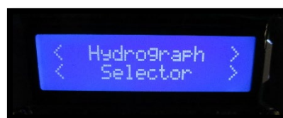
Figure 9.5 Menu Screens on the K500 Controller
